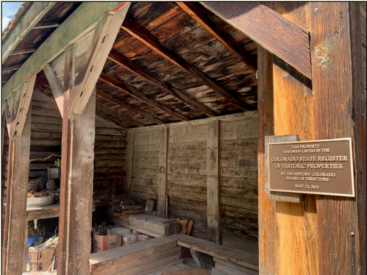
View of the interior of the Denver & Rio Grande Western Railroad Passenger Shelter showing the back and side walls that are covered with numerous historic inscriptions including individuals' names, dates, place names, descriptions of activities undertaken in the area, and drawings of humans and animals. Photo by Kim Marvel.
